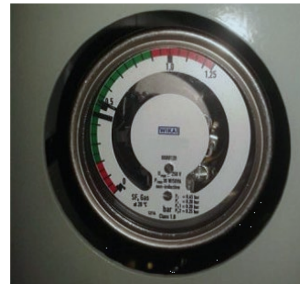
Gas Pressure Indicator
