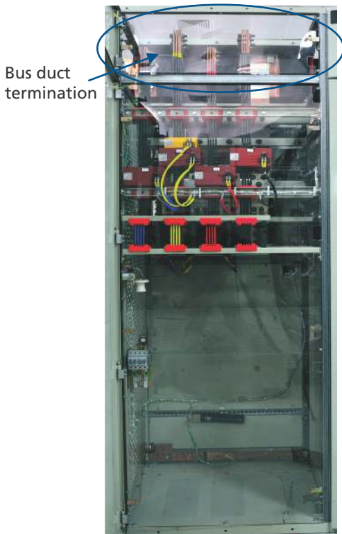
Figure 27 - Top Busduct termination
