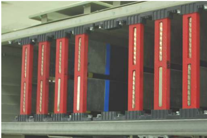
Figure 3 - Double Deck arrangement of busbars
