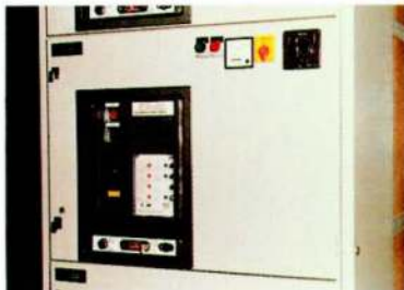
Compartment housing ACB with microprocessor based release.
