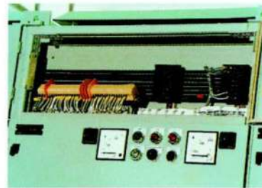
Auxiliary busbar arrangement and interpanel wire terminations.
