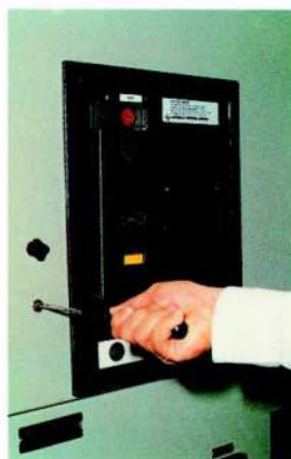
Door interlock defeat facility
