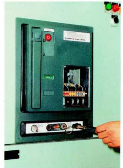
Storage slot for racking handle.
