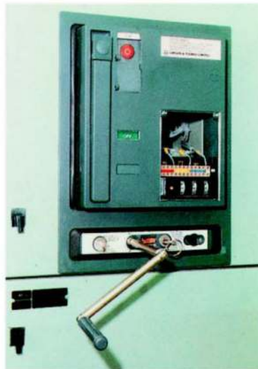
Breaker in 'Test Position', with the door closed.
