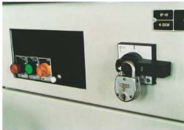
Padlocking for power switch
