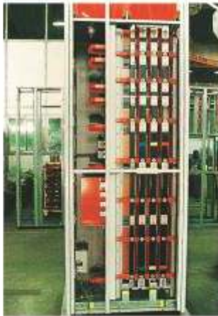
Completely sleeved busbars & droppers
