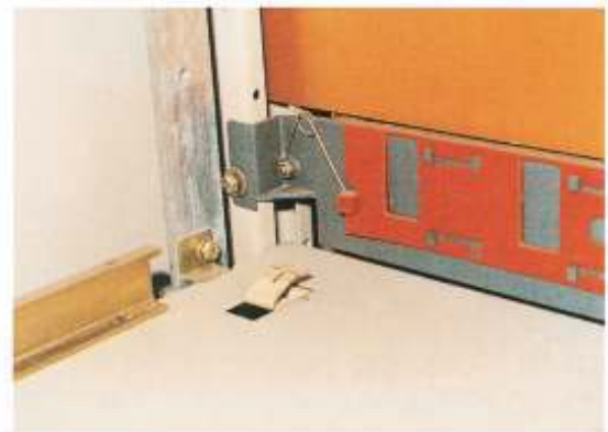
Earthing of chassis is achieved through scraping earth
