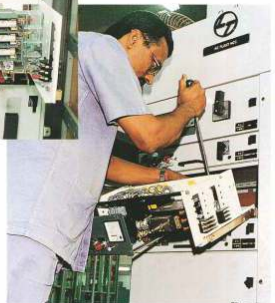
Maintenance being carried out on a 200 mm module
