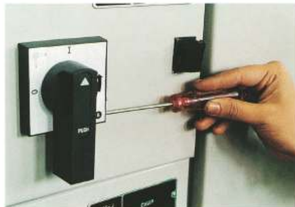
Door interlock defeat facility
