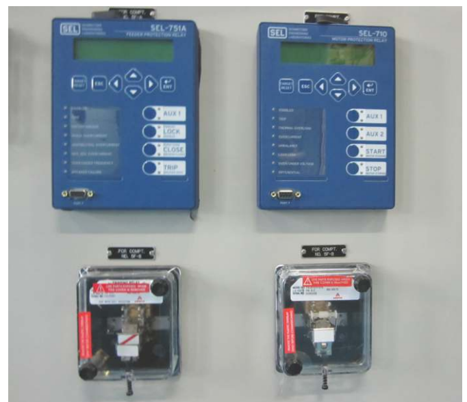
Figure 47 - Relay Mounting on Panel
