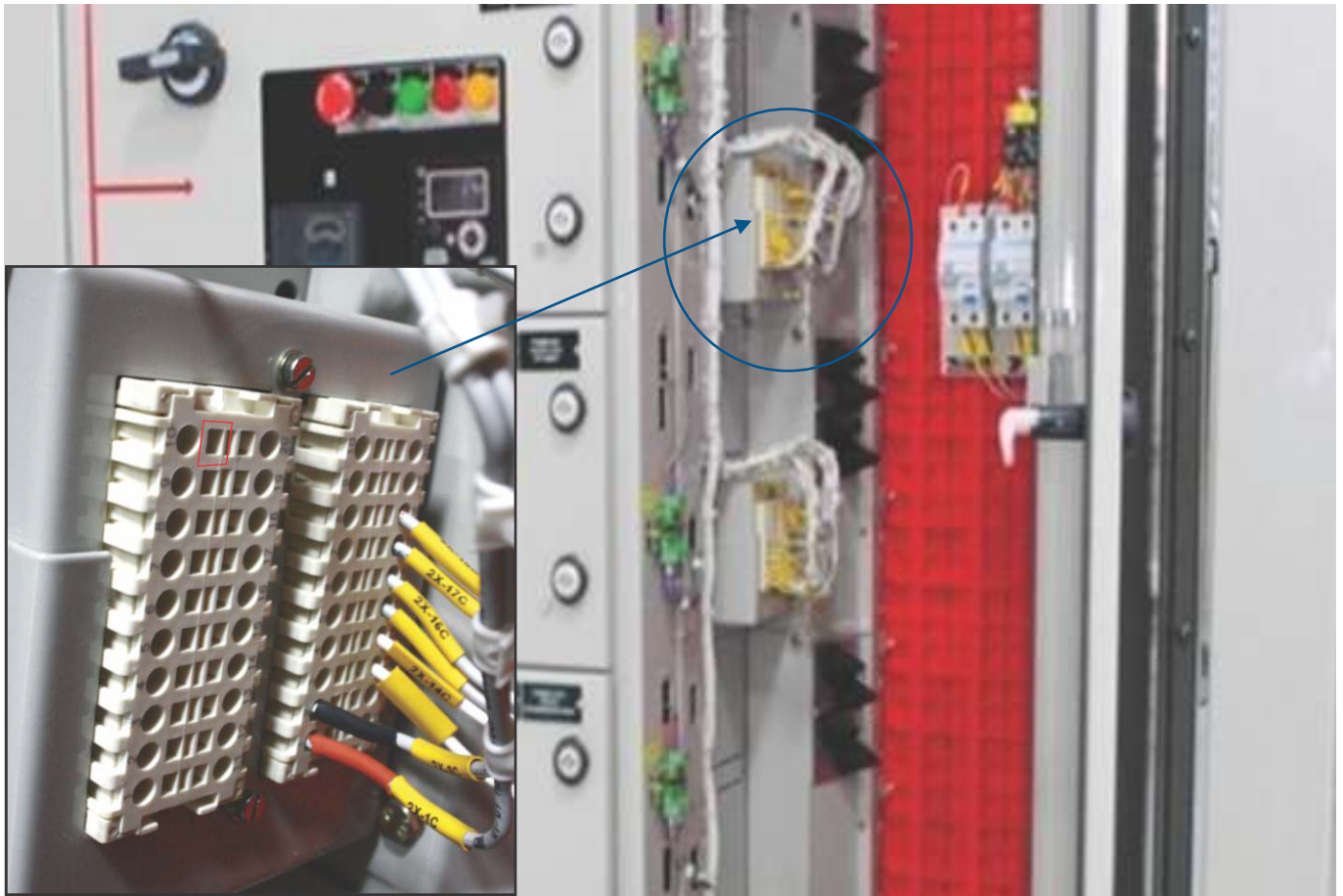
Figure 45 - Control Cable terminals
