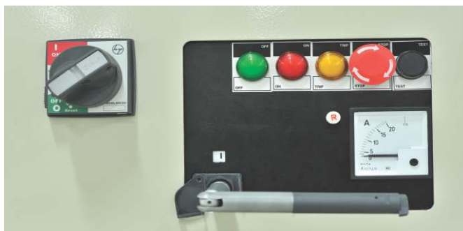
Figure 56 - Full width module in Isolated position
